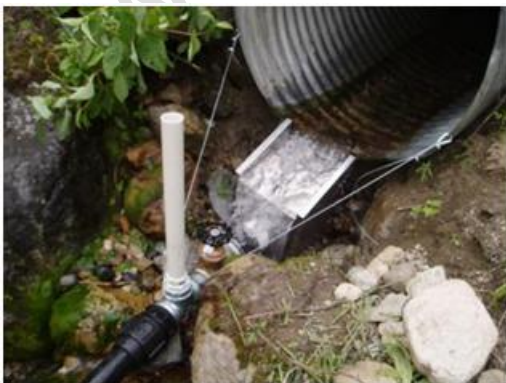
Commercial intake on road culvert
