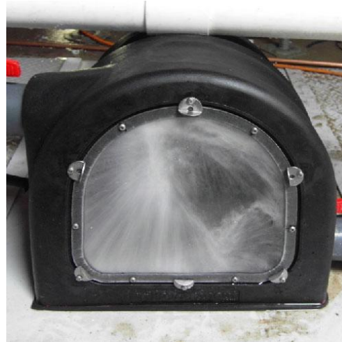
Top and bottom jet exhaust water is bouncing back towards the jet, turbine is running slow, a little more packing is needed
